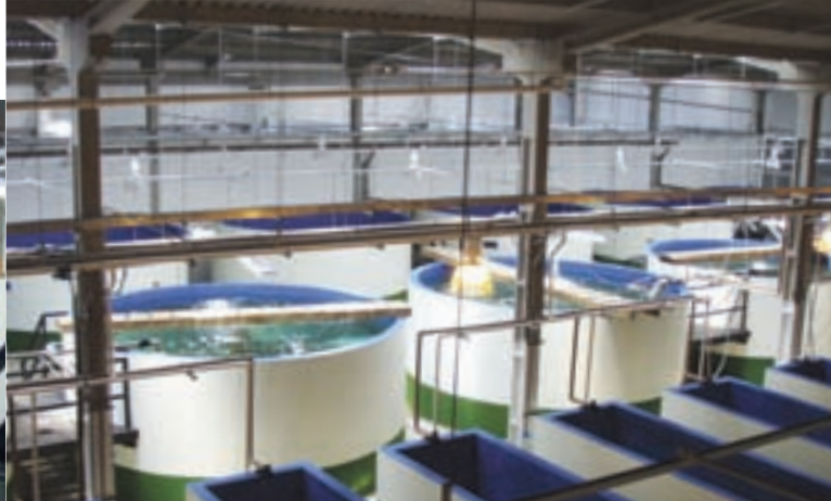
The state-of-the-art hatchery at the National Laboratory of Aquaculture in Brazil incorporates a large-scale broodstock facility and associated infrastructure to support fingerling production for the country's growing cobia industry.
